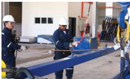
Maintenance of wireline surface equipment
