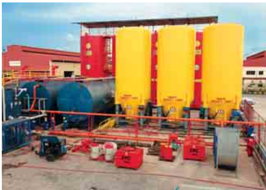
Liquid Mud Plant
