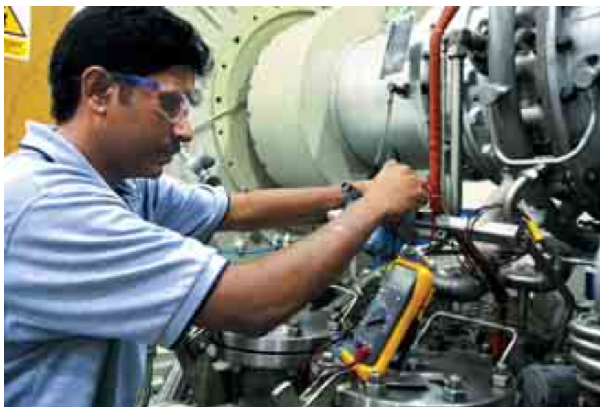
System testing on a gas turbine unit at Turboservices: Solar Turbines Integrated Service Centre.
