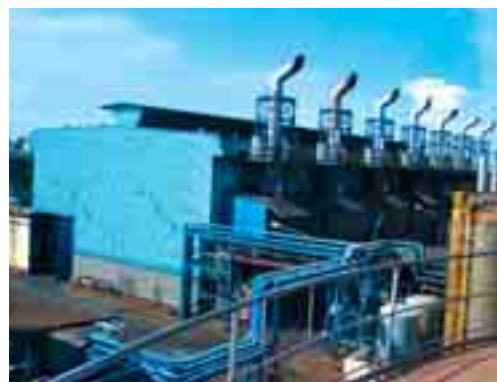
CUPL Power Plant, Cambodia.
